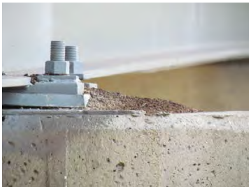
Photo 5: Guano deposit on pier, obscuring structural features.
