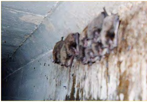
Photo 1: Bats hanging from cracks along Support beams
