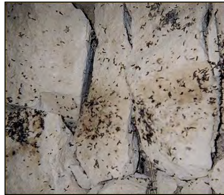
Photo 6: Bat Guano on Riprap
