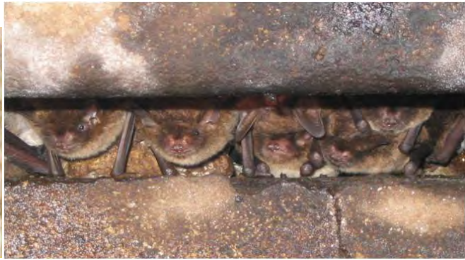
Photo 2: Visible bats within an expansion joint
