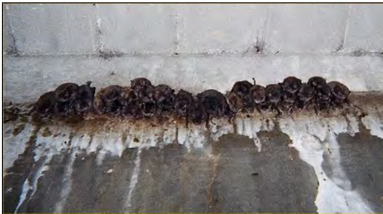
Photo 11: Bats Roosting & Associated Staining
