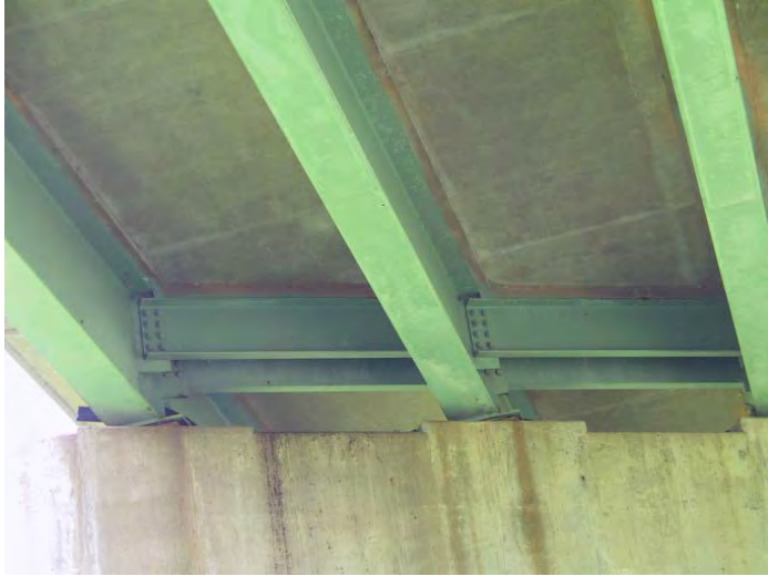
Photo 10: Guano staining on side of pier
